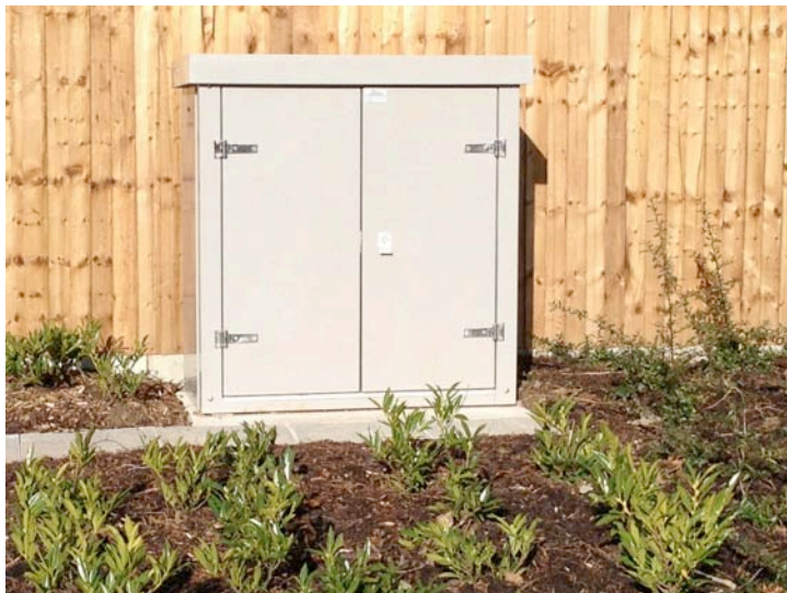
Example of cabinet for housing controls:
